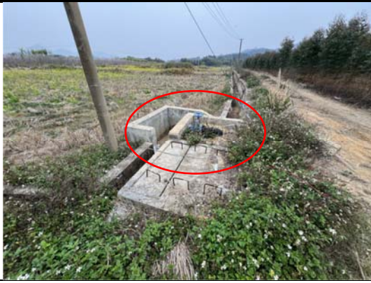
北部灌区放水闸阀
